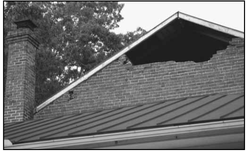
More earthquake damage: a hole in the back wall of the sanctuary of Gilboa CC.
